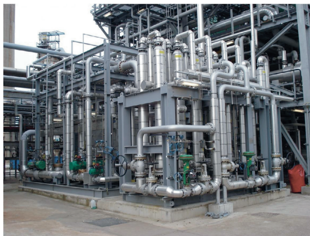
Figure 3. A PRISM ® hydrogen recovery membrane installed at a refinery. Hydrogen recovery membranes can return hydrogen streams of up to 98% and in some cases 99.9% hydrogen purity.
