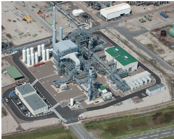
Figure 2. The newly installed hydrogen facility at ExxonMobil in Rotterdam improved energy efficiency over the previous hydrogen supply by over 15%. It also lowered CO 2 emissions by over 200 000 tpy.
