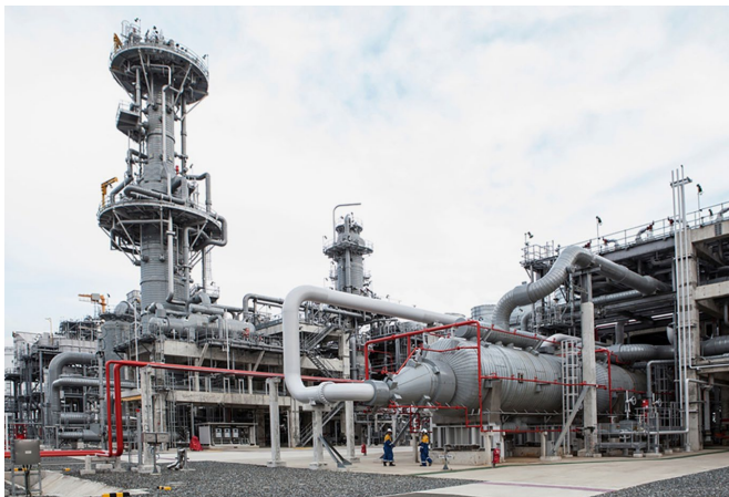
Donggi-Senoro LNG, Indonesia utilizes Air Products' propane pre-cooled mixed refrigerant (AP-C3MR™) LNG Process.
